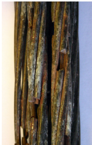
Figure: Broken tension wires.
